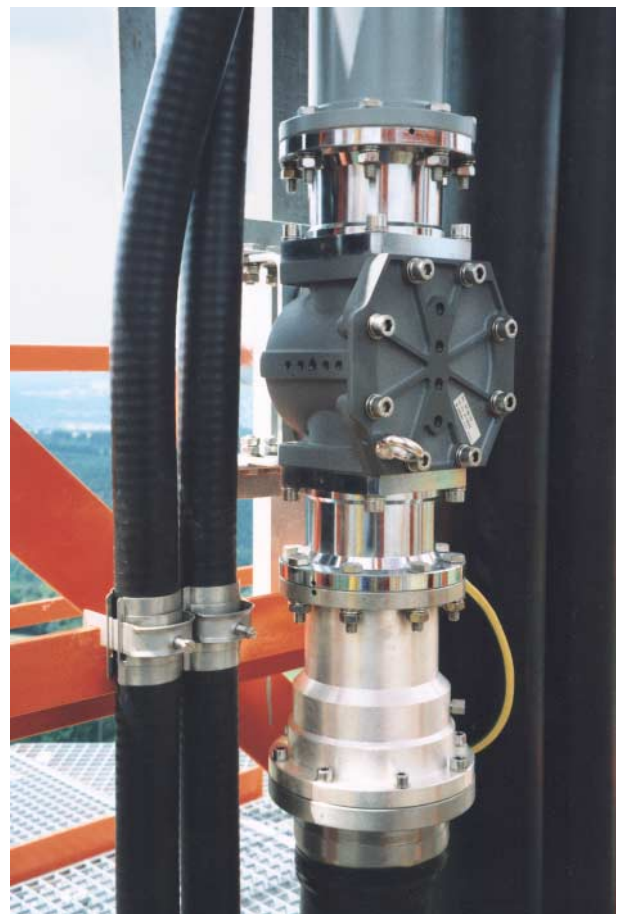
Measuring link in a cable run
